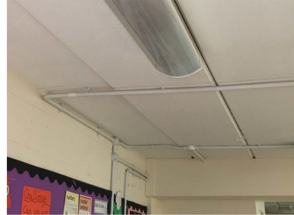
Figure 10: Example of deflected RAAC panel
