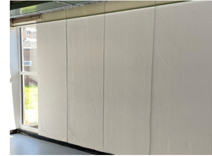
Figure 5: Example of RAAC on internal wall face
